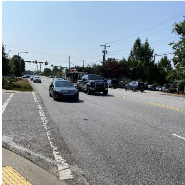
Existing pavement markings worn out
