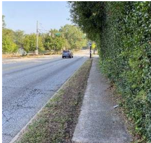
Overgrown Vegetation near Blythe Drive
