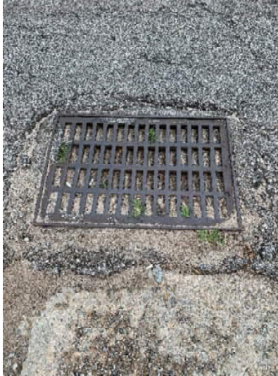
Catch Basin Blocked with Silt
