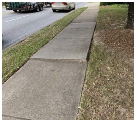
Uneven Concrete Sidewalk
